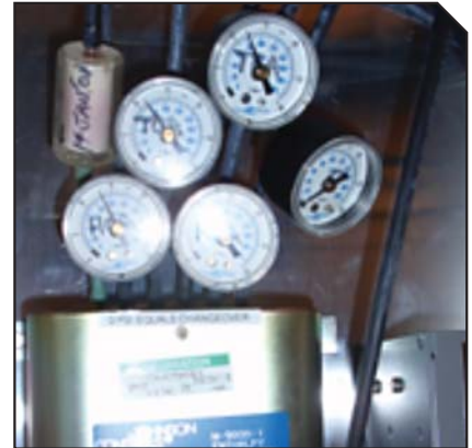
FIGURE 7. Example of existing pneumatic controls.
